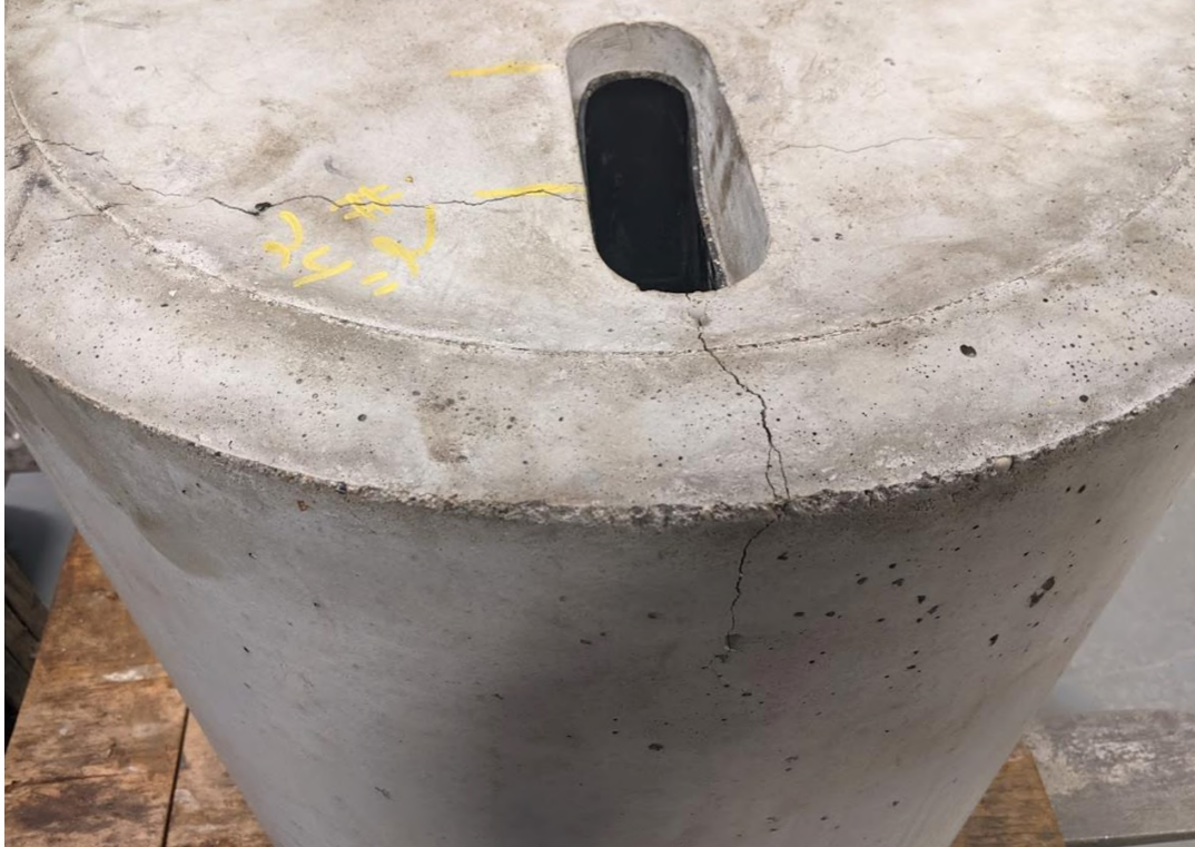
Figure 4: Typical Cracking Pattern
